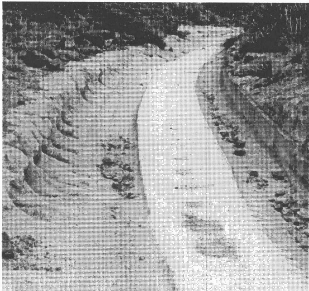
These deep ruts, found in solid rock, were made by ore wagons going through Kingman, AZ. photo by Robert Lee
