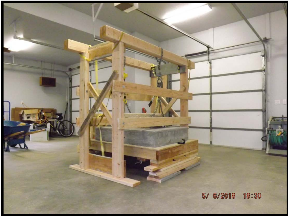
Gantry for lifting the repaired marker and the new concrete base off of the cart
